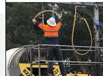
Pictured: Concrete Truck Driver at Slumpstand with ME4T-PC with CMM25 mag c/w pulse re-transmission to batchroom UIC to PLC input
